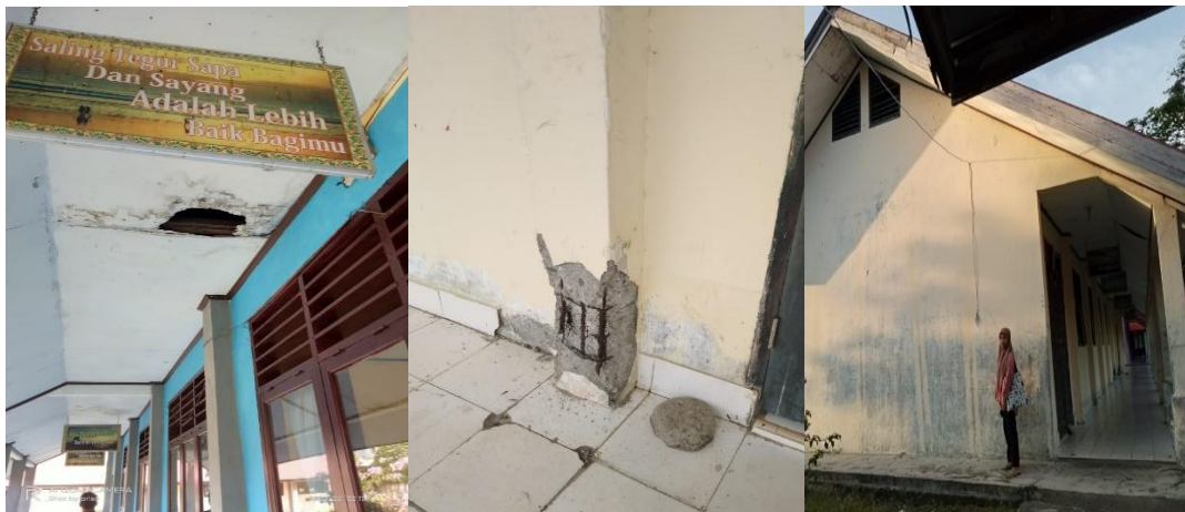
Figure 1. Damage elements of the school of SMPN 2 Meulaboh
