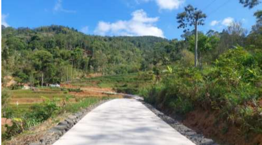
Figure 4. Concrete condition in normal sunlight Source : Personal documents
