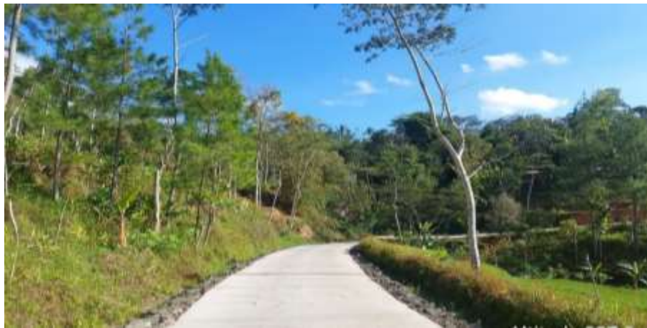
Figure 5. Concrete condition with abnormal sunlight
