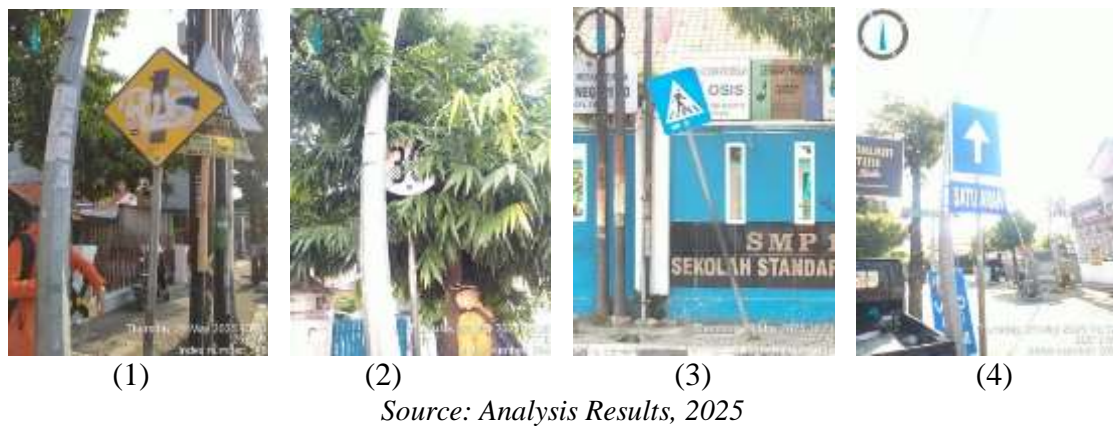
Figure 3. (1) Intersection warning sign covered with spray paint (2) Speed limit sign obstructed by vegetation (3) Crosswalk sign pole is tilted (4) One-way implementation sign
