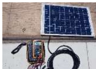
Gambar 12. Pengujian panel & switching relay
