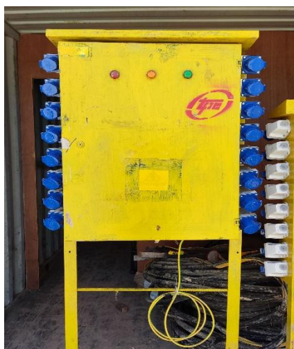
Gambar 3. Sub Distribution Panel (SDP)
